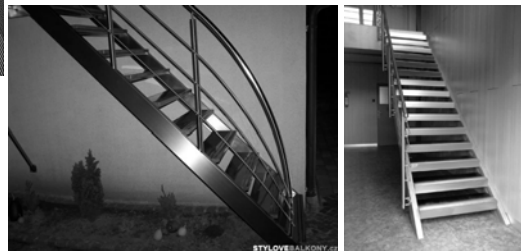
Interior stainless steel elements
