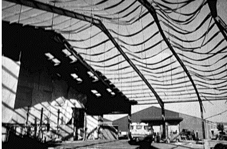
Fire safe structure – no collapse was observed, people were not in danger when escaping / fighting with fire
