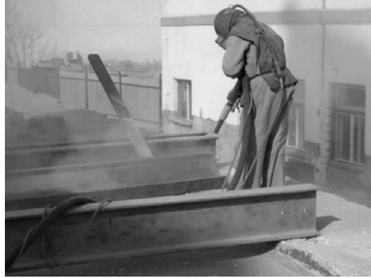
Grit blasting of steel beams on-site suitable for repairing of existing structures
